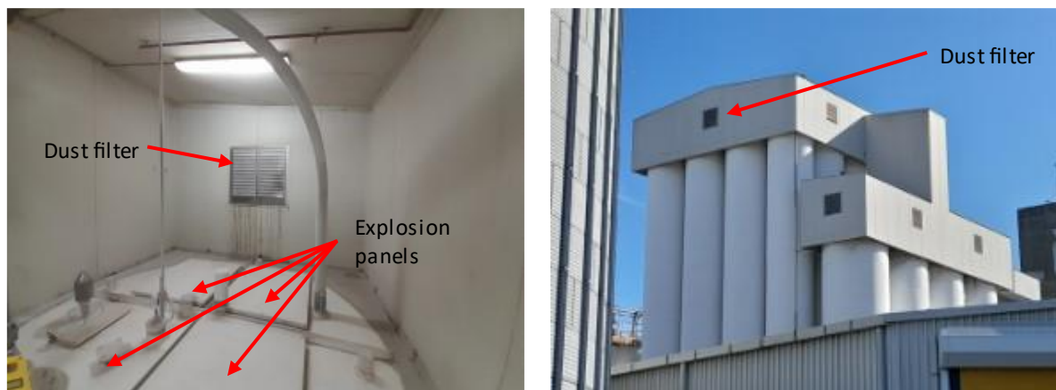
Figure 5.10: Explosion panels and passive dust filters in explosion panel room above finished product silos.
