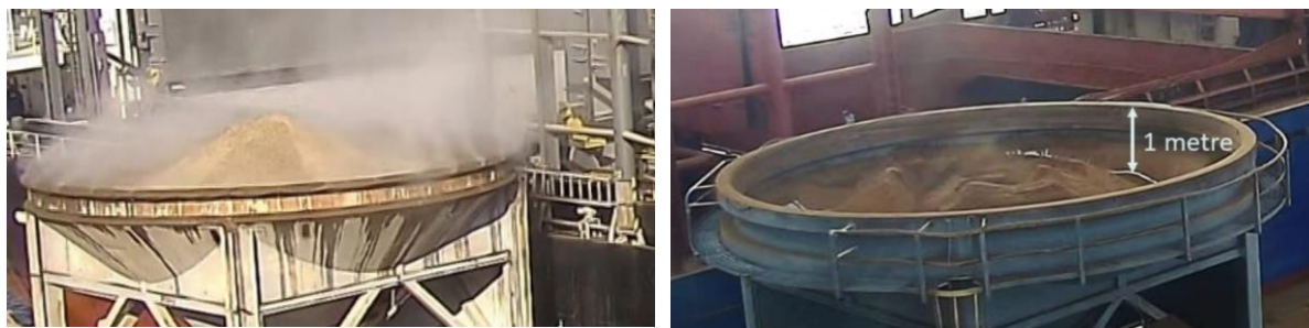
Figure 5.5: Left: Maximum fill height for hopper with grizzly. Note this picture shows a hopper with misting sprays. Misting spray are not mandatory. Right: Maximum fill height for hopper without grizzly.
