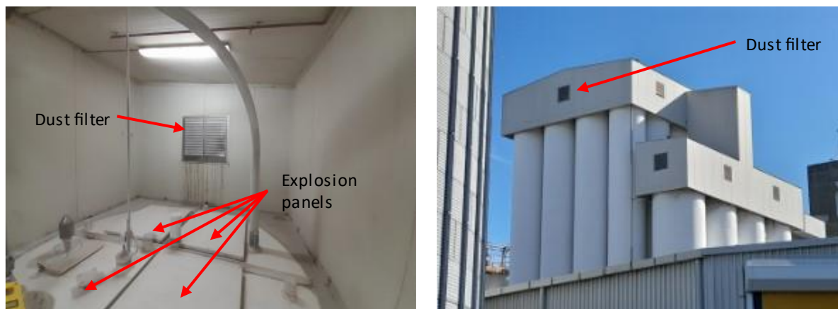
Figure 5.10: Explosion panels and passive dust filters in explosion panel room above finished product silos.
