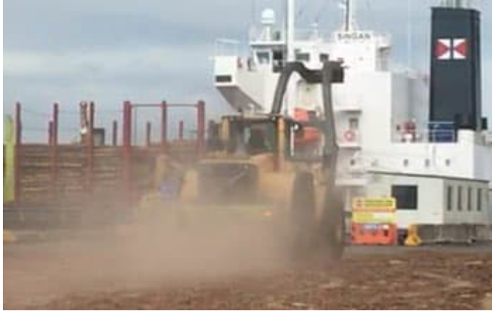
Figure 1: Example of excessive visible airborne dust
